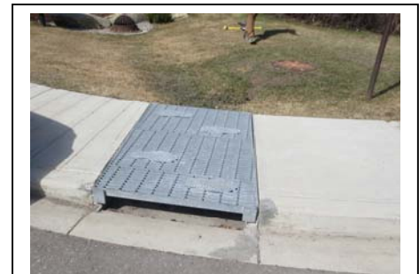
Photo 2-3: Curb cut leading to bioretention area through sidewalk with a grated top, Marlowe Place, Calgary, AB
